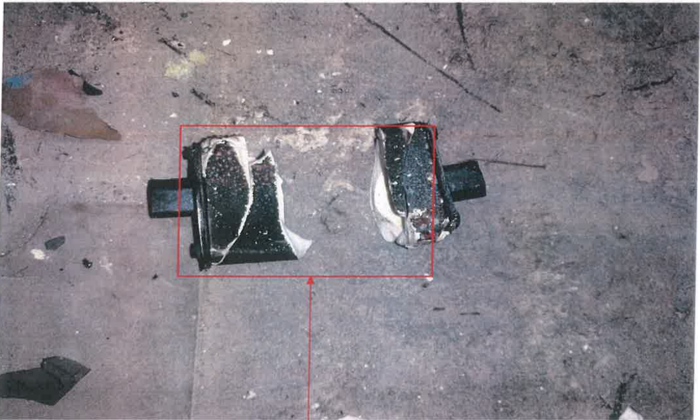
Broken HRC (High Rupturing Capacity) Fuse
