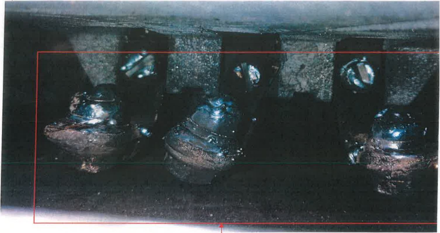
Melted Terminals of Electrical Module
